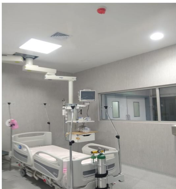
Figura 64 Luminarias Agat Clean Led 36 W 5200 Lm 840/600X600 PLX
