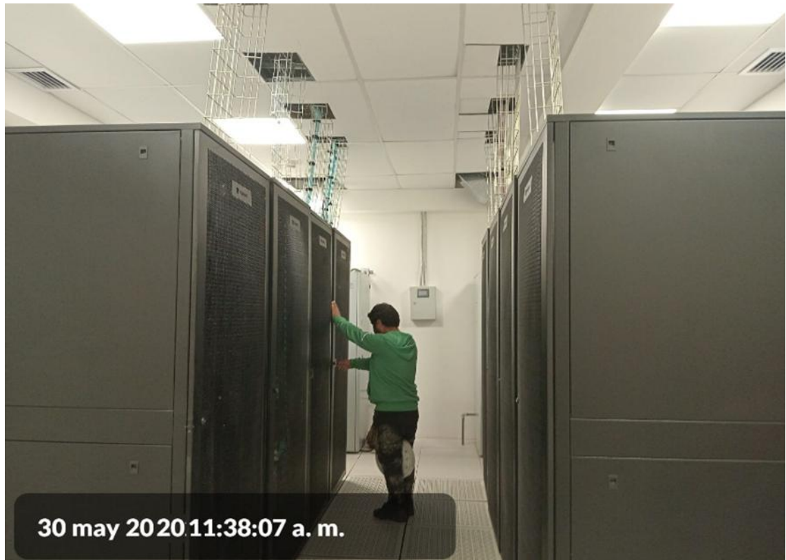
Figura 30: Data center del hospital regional de cañete
