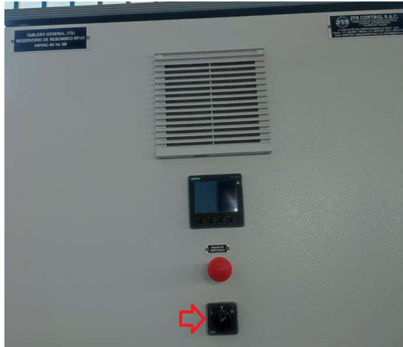
Selector LoR (Local – 0 – Remoto) del Tablero General
