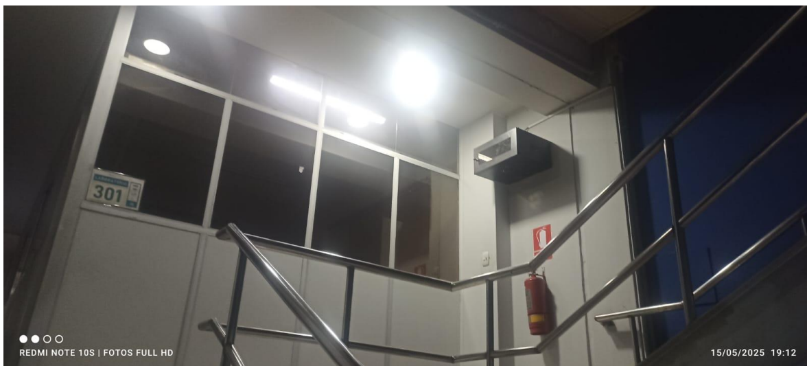
Fig. 70. Gabinete de pared Switch PoE
